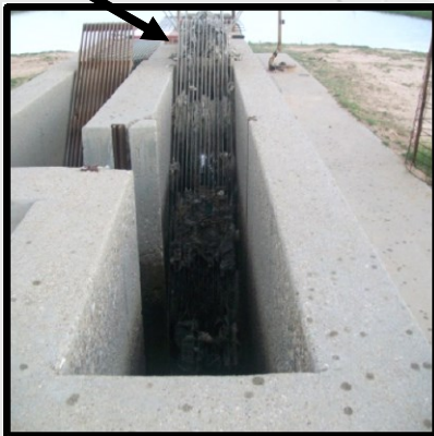
Headworks and bar screen
